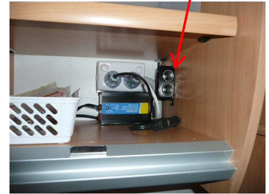
Added 12v outlet to connect inverter to power DVD player [when 240v AC not available] [located inside overhead cupboard near exist- ing PP used by DVD player]
