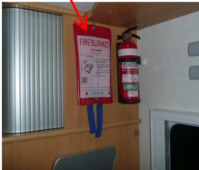
Added fire blanket [near door]
